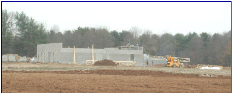
The photo (above) was taken on Veteran's Day (11/11/04) and shows the progress being made on Tasty Blend's new office.
