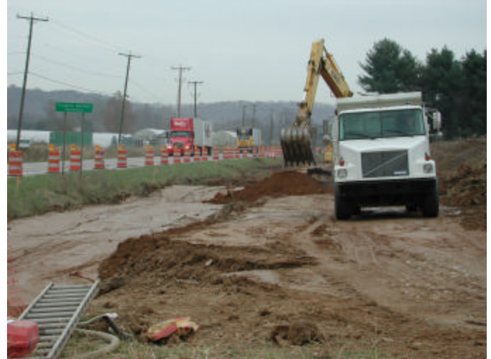
A truck finishes dumping another load of fill dirt alongside U.S. Route 35, as contractors work to install turn lanes.
